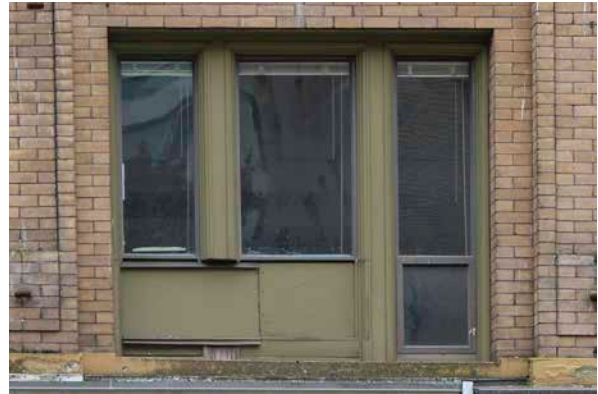
Front façade window with original wood frame and mullions, but with non-original sashes and glazing. Portion of mullion has been removed, and two lower sashes are boarded over. (Donald Luxton & Associates)
