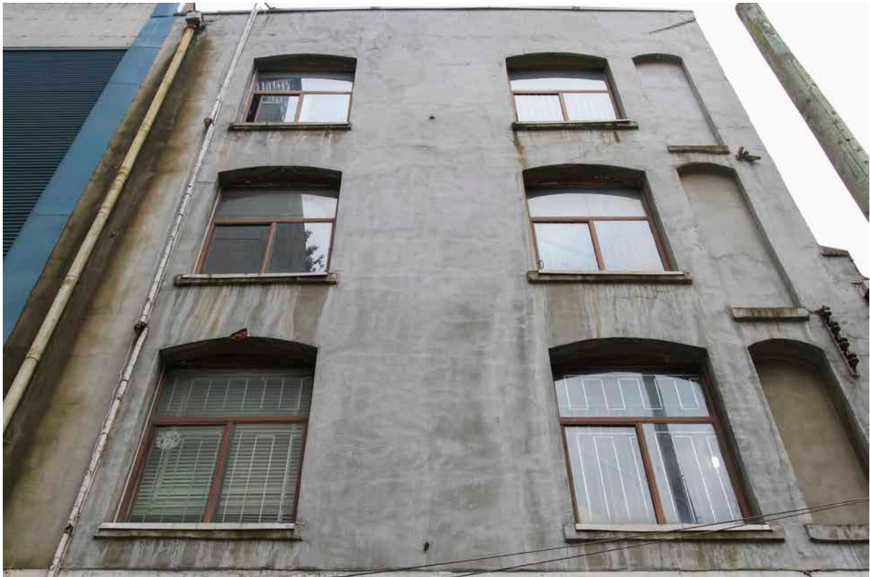
View of the rear façade of the Allen Rooms with brick structure covered in a rendered. (Donald Luxton & Associates)
