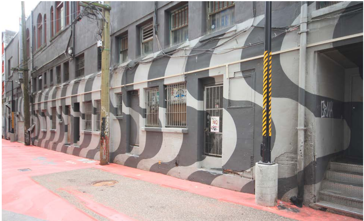
Rear façade of Commodore Ballroom showing parged brickwork with parging failing at right.
