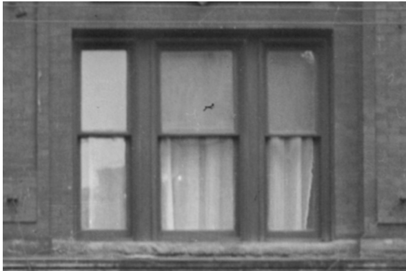
Detail of the original wood window assemblies on the front façade of the Allen Rooms in 1950. (Artray; Vancouver Public Library 81449)
