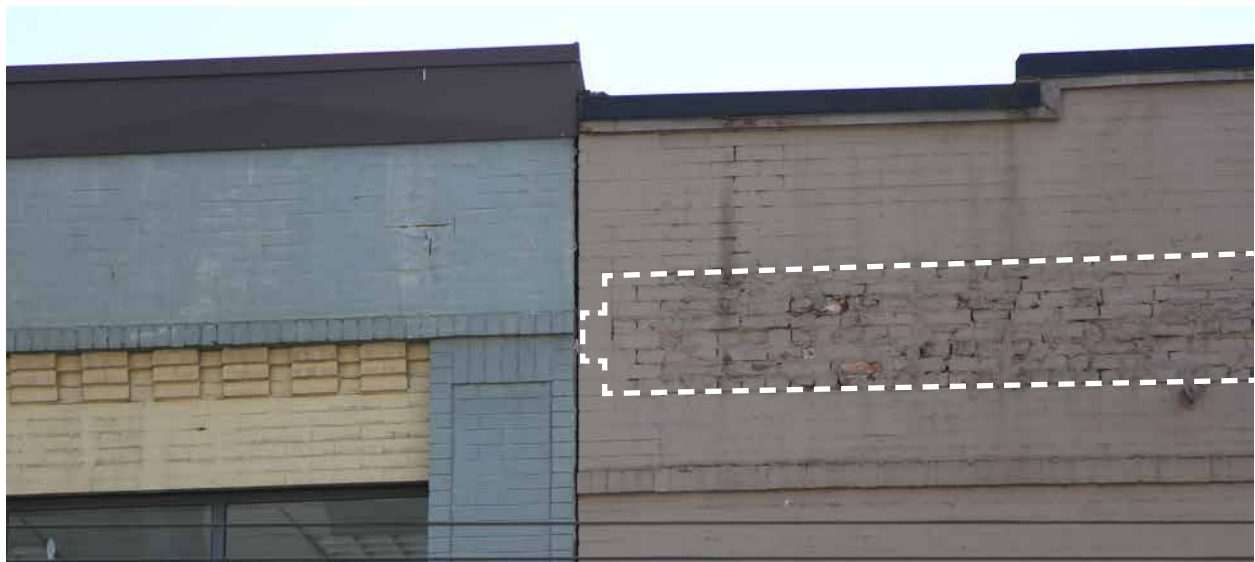
Detailed view of parapet wall corner showing outline of missing cornice and later added cap flashing as it appeared in March 2021. (Donald Luxton & Associates)
