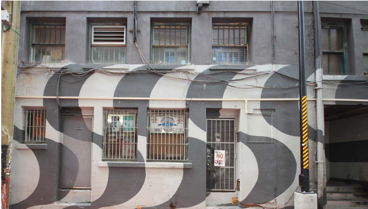
Rear façade of Commodore Ballroom with metal hung windows. Some of the windows have been altered, contain broken glass, openings filled in, or have bars installed in the window openings.
