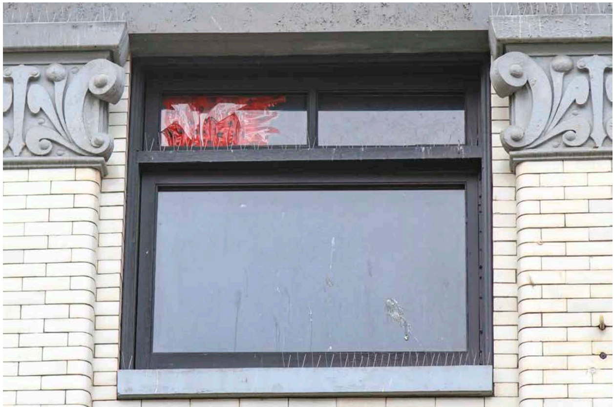
Detail of a typical, original wood window assembly on the front elevation of the Norfolk Rooms, July 2021. The single-lite sash is operable, featuring a vertical central pivot mechanism. (Donald Luxton & Associates)
