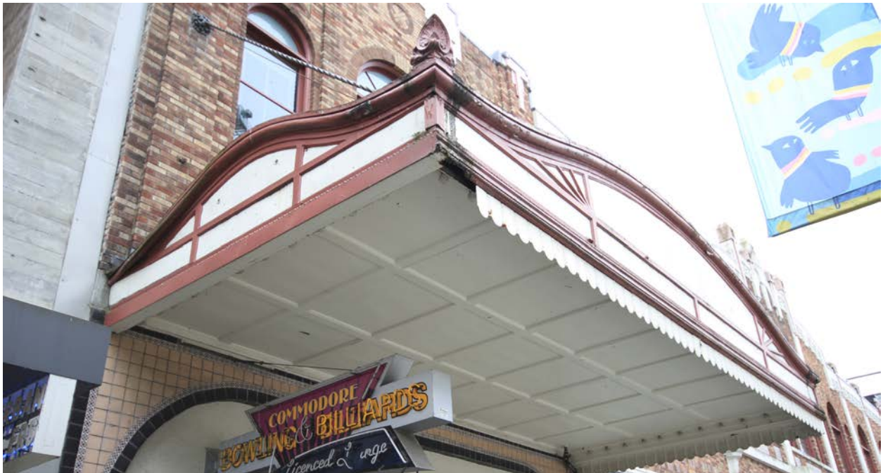
Below: Extant canopy at north end of the Commodore Ballroom with missing cresting elements and portion of detailing below the canopy missing. Corrosion and staining is also evident at corners of canopy.
