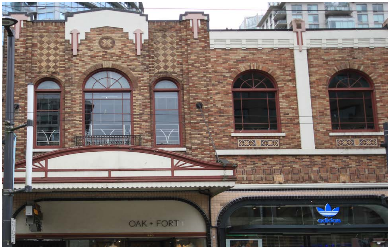
Single and triple assembly windows of the second floor of the front façade. Original wood jambs and sashes are largely intact; however, some sashes and glazing have been replaced.
