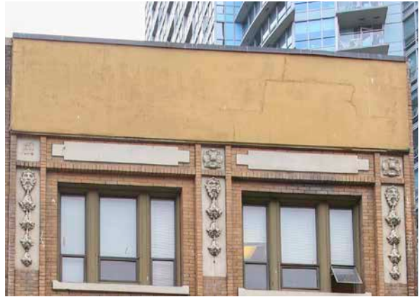
Parapet with missing cornice since c.1949. Currently the parapet features a solid cement render finish with signs of staining, cracking, and paint peeling. (Donald Luxton & Associates)
