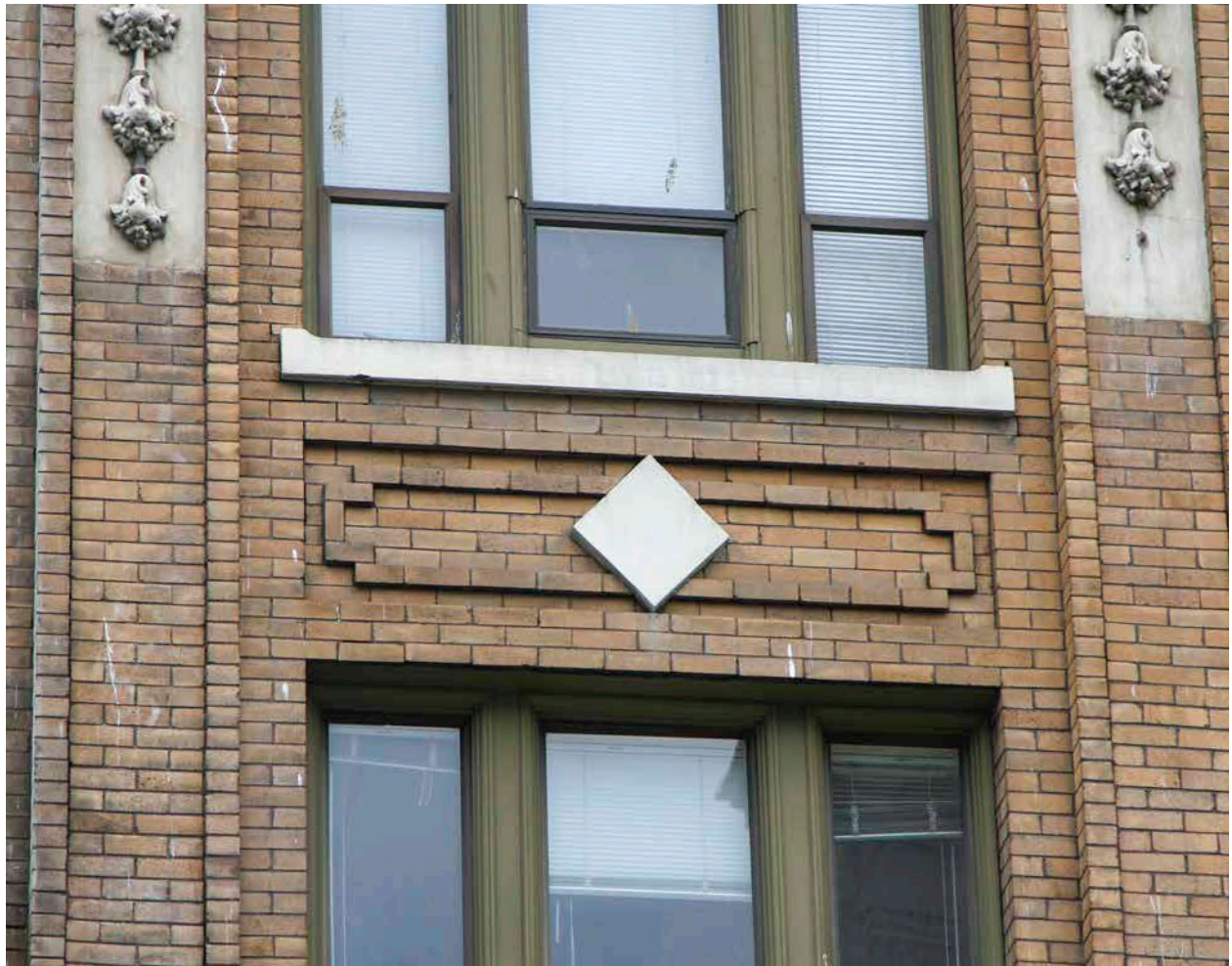
Front façade showing brown-coloured brick in running bond and brick-bordered end pilaster. Spandrel panels feature decorative borders, and ornamental precast concrete rhombus in the center with matching concrete window sills above. (Donald Luxton & Associates)
