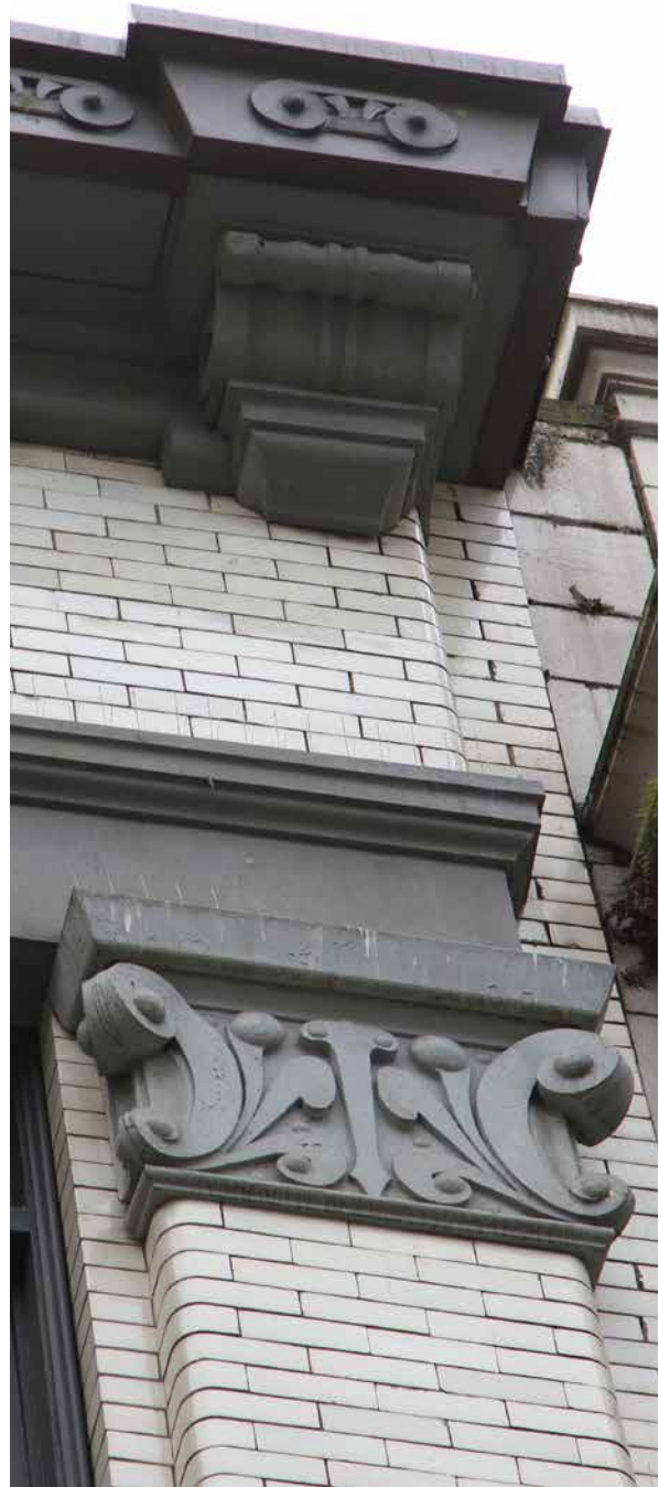
Detail of the Corinthian capital; lintel band; and cornice of the Norfolk Rooms, July 2021. (Donald Luxton & Associates)
