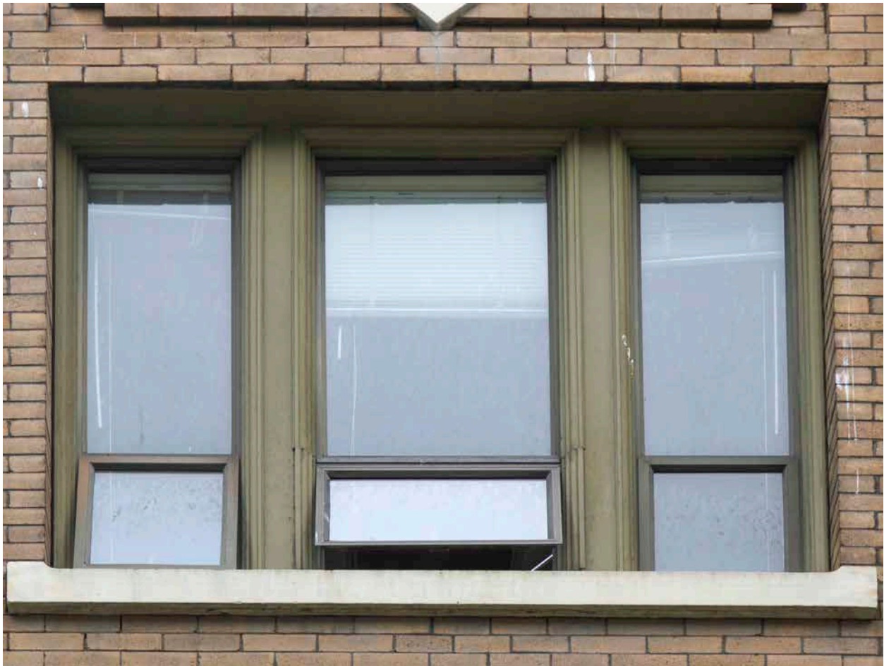
Front façade window with original wood frame and mullions, but with non-original sashes and glazing. (Donald Luxton & Associates)
