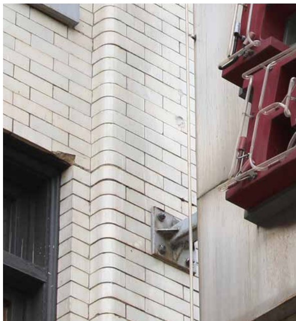
Damage, discolouration, and past patching visible on the face brick of the front façade, July 2021. (Donald Luxton & Associates)
