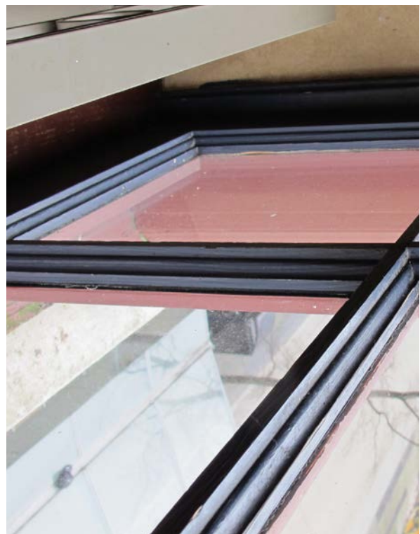
Top: Original sash spool of second floor double hung window. Hung windows were changed to two-lite fixed sash. Bottom: Original multi-lite wood sash window from interior.
