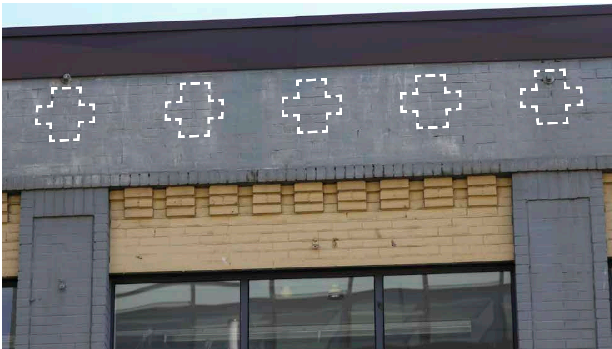
Detail of brickwork along the second storey of Granville Street façade, July 2021. Original, decorative brickwork (outlined above) is evident but obscured by paint. (Donald Luxton & Associates)
