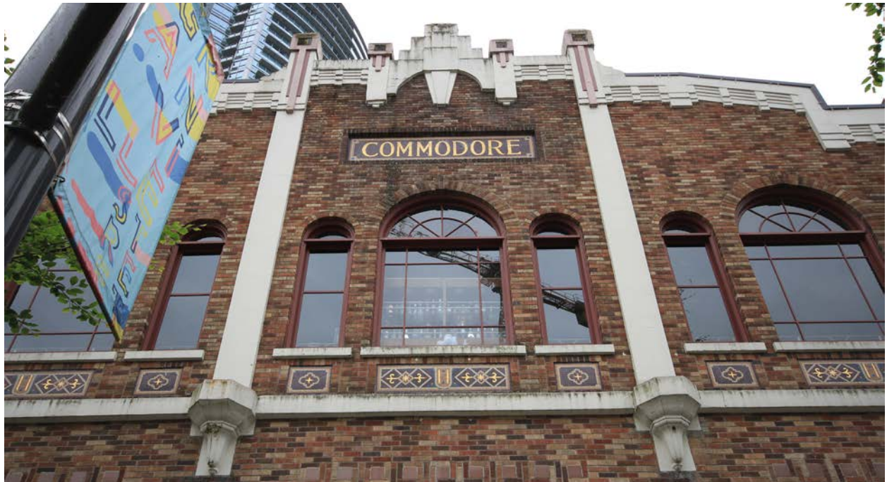
Central parged ziggurat and geometric detailing among the Commodore Ballroom's parapet. Pilasters with geometric details. Note staining on brickwork around 'COMMODORE' sign band and on horizontal sills.
