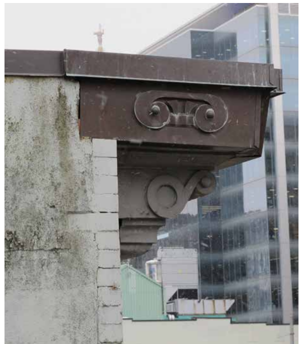
Detail of the cap flashing on the parapet and cornice of the Norfolk Rooms, July 2021. (Donald Luxton & Associates)
