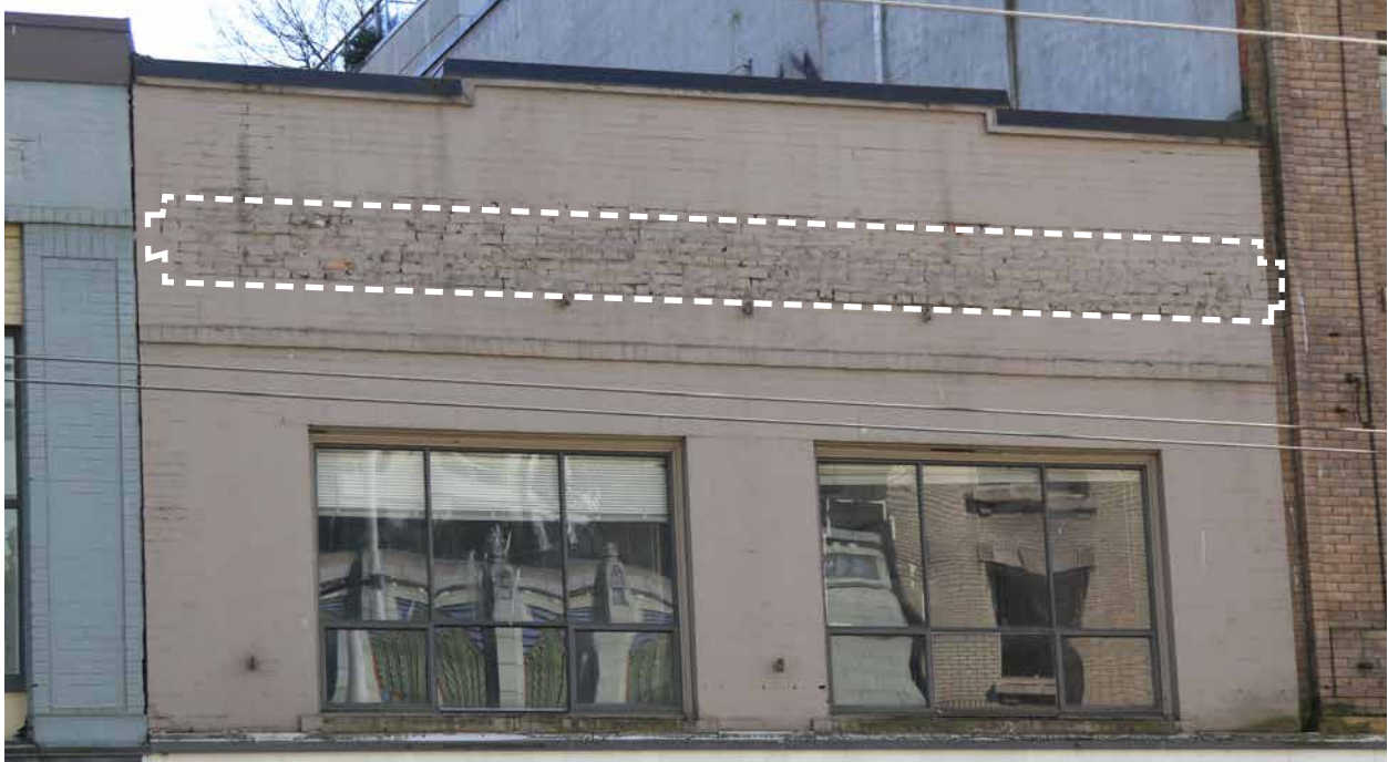
View of the upper floor of the front façade from Granville Street as it appeared in March 2021. Note outline of missing cornice. (Donald Luxton & Associates)
