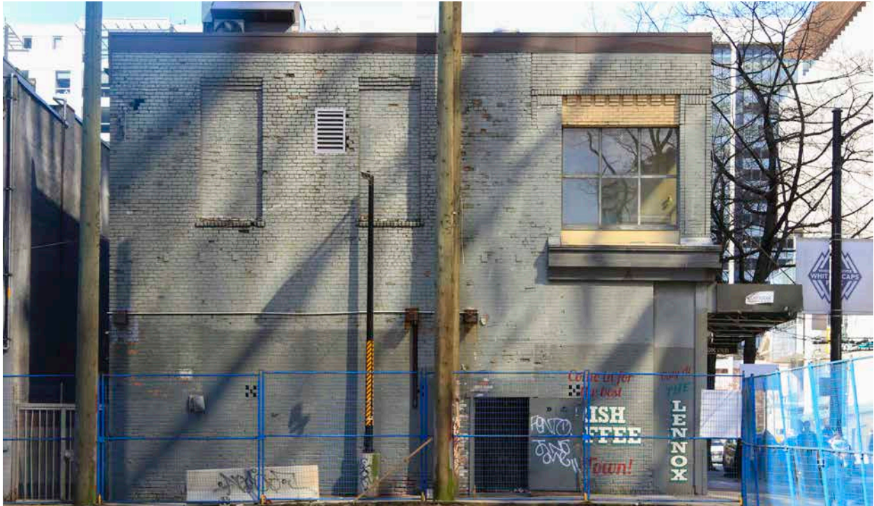
View of the Service Building's rear façade as it appeared in July 2021. (Donald Luxton & Associates)
