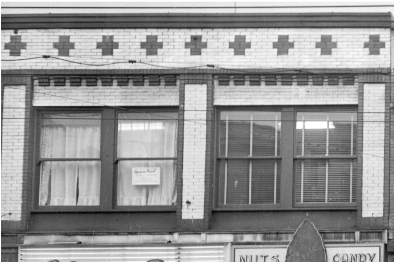
View of original double assembly wood sash windows as they appeared in 1950 along the Granville Street façade. (Artray, Vancouver Public Library 81449)
