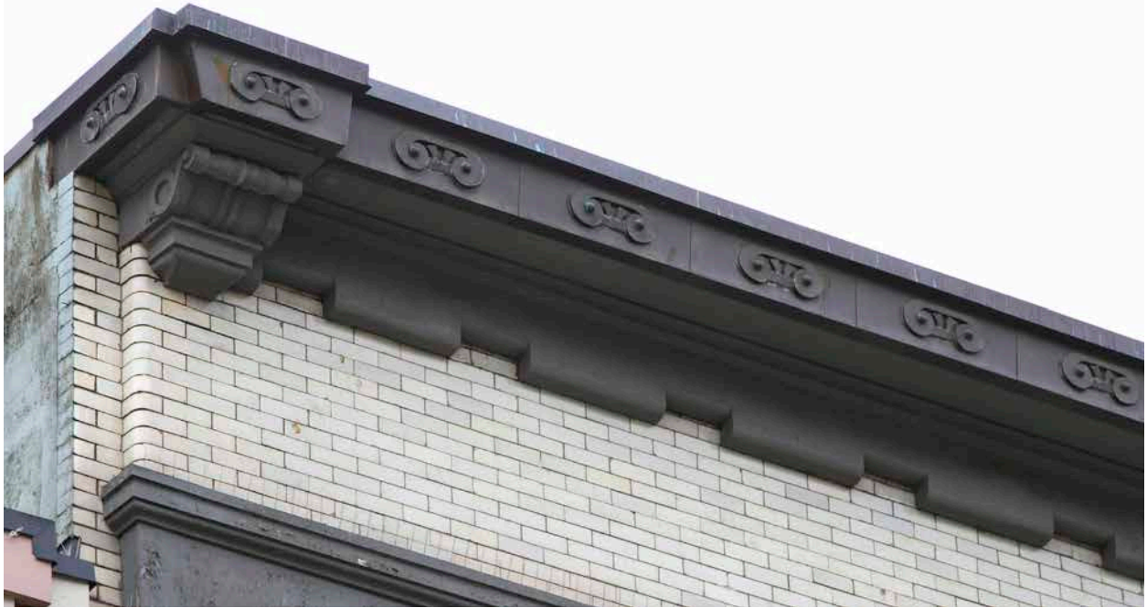
Detail of the parapet cornice along the front façade of the Norfolk Rooms, July 2021. (Donald Luxton & Associates)
