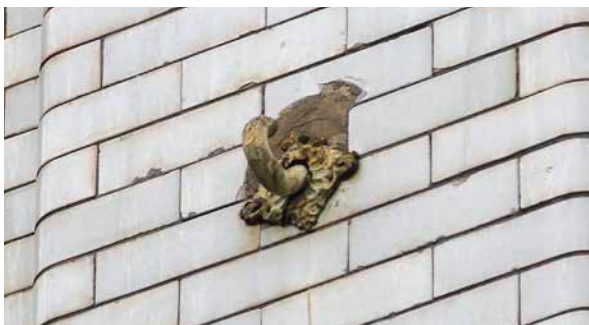
Detail of one of two decorative anchors installed in 1924 to support the Commodore Cafe marquee, July 2021. (Donald Luxton & Associates)
