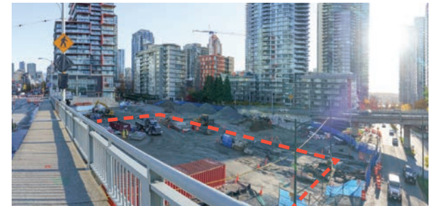
The site with roadworks underway, from the north end of the Granville Bridge
