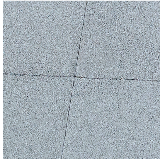
DURASAFE RUBBER TILES AT FITNESS AMENITY
