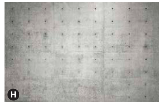
H Concrete Wall against the lot line which defines the property boundary.
