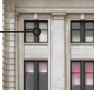
DARK GREEN METAL PANEL LOCATION - WINDOW FRAMES, MULLIONS, LINTELS, AND CANOPY STRUCTURE AT LEVEL 1
